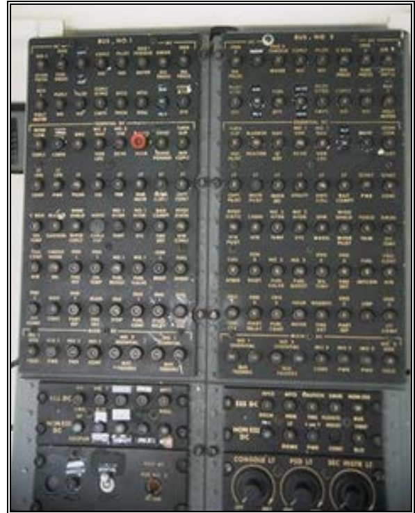
Figure 3-27 Aft Circuit Breaker Panel
